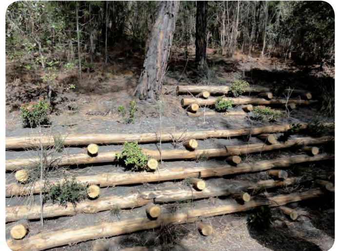
Photo 2.17: This small ecological engineering works are done to stabilise eroded slopes. They combine the use of local wood logs and the revegetation with woody species that have been carefully selected. It is important to respect the proposed standards regarding the logs dimension as well as the plantation density to guarantee the sustainability and the efficiency of the works.
