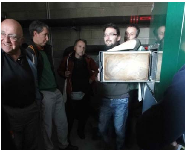
Photo 9: Boiler with a thermal output of 350 kilowatts.
