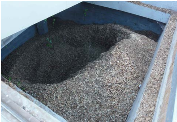
Photo 10: Stock of wood chips for delivery trucks, directly supplying the burner through a feeder screw.
